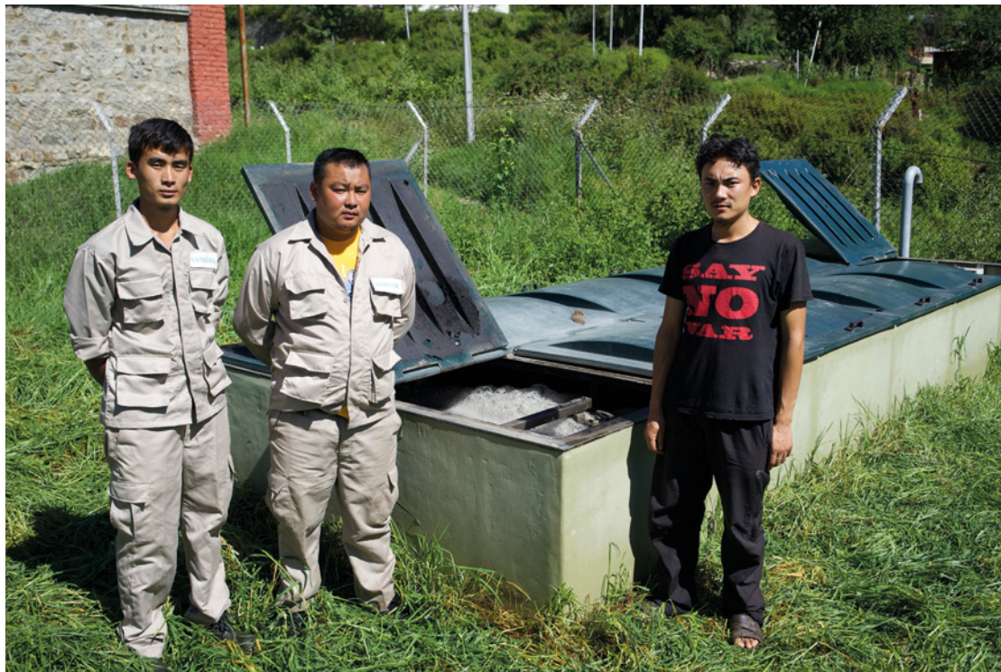
Sangsel Eco Trade technicians and service staff in front of Ecoline wastewater treatment plant in Thimphu
