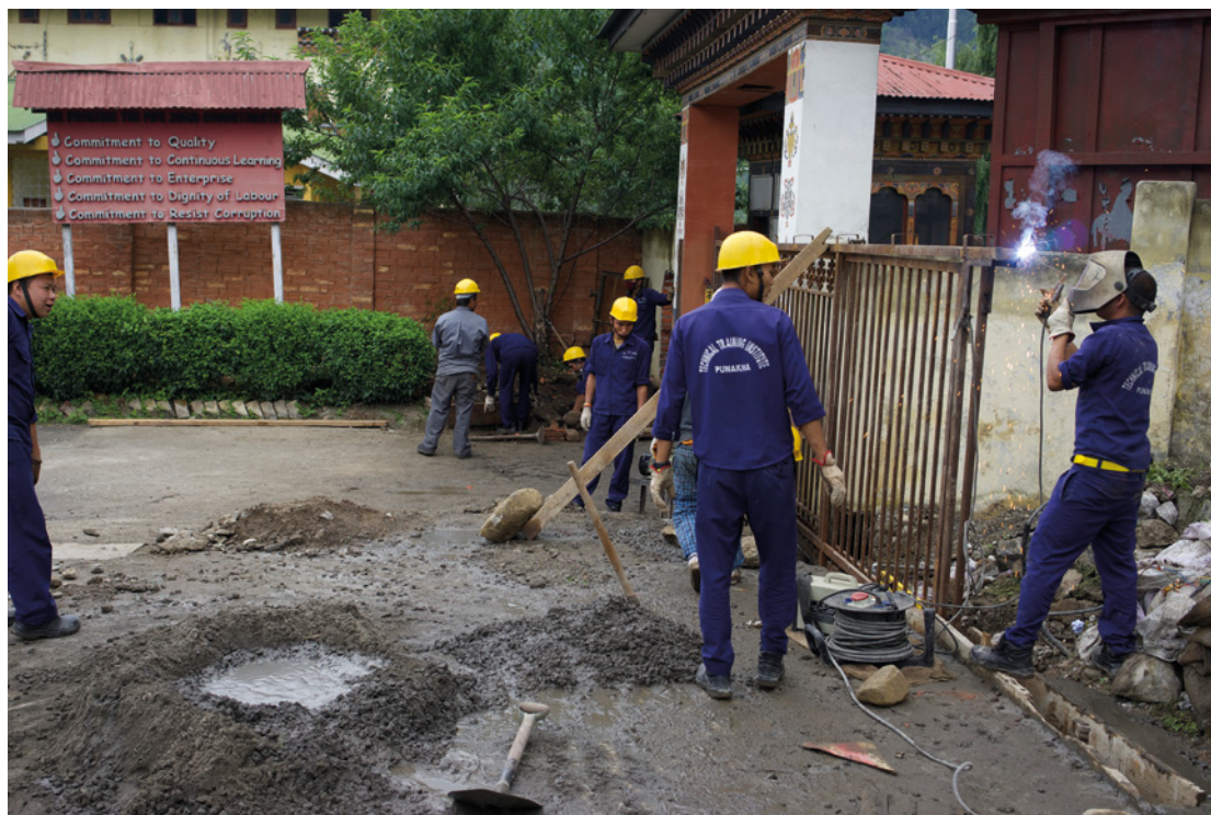
Students from Technical Training Institute in Punakha makes renovation at the Ministry
