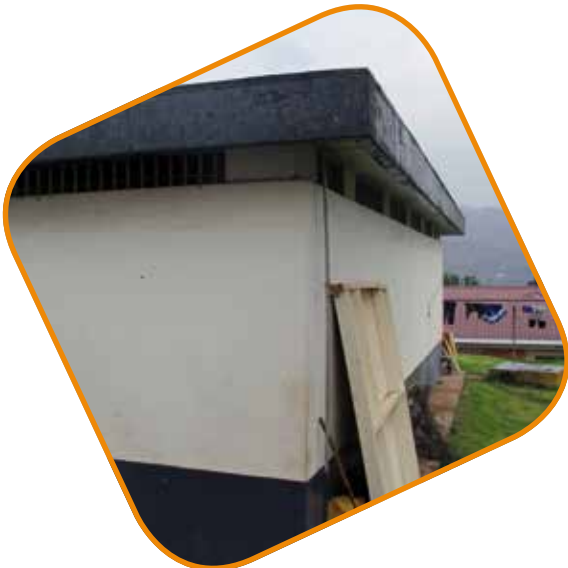
Photo: Structure of old mental health units in regional hospitals, unit in Kabale hospital, October 2013. © MDAC.
